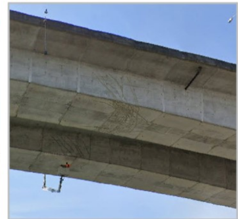
C Cracking in bridge center
